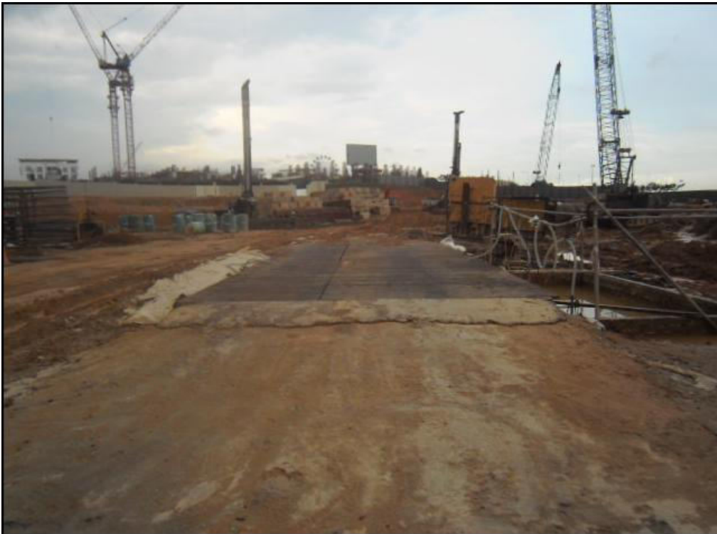
Wash trough provided at site
